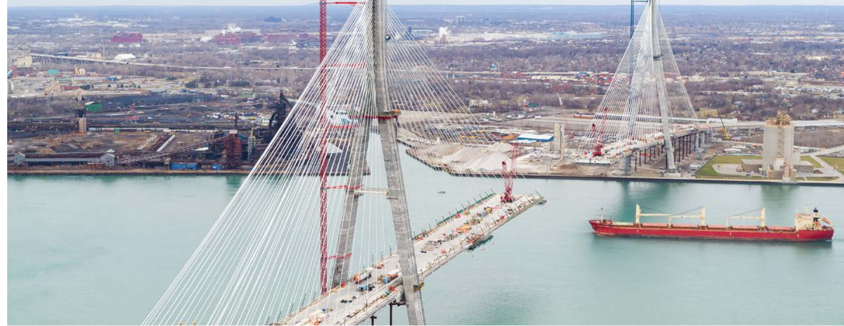
▲ The Gordie Howe International Bridge project in Windsor, Ontario, Canada. / Progress December 2023 / Image credit: Gordie Howe Inter. Bridge
