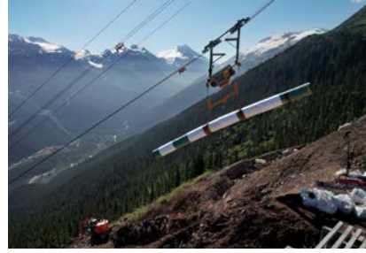
▲ Coastal GasLink installed approximately 1,400 meters of pipe this summer across what the project calls Cable Crane Hill in Section 8.
